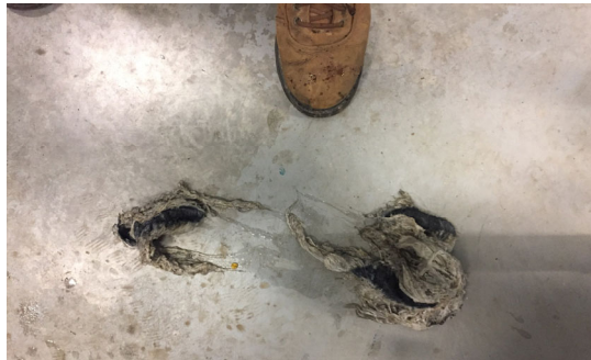
(Picture of wipes that clogged the pumps)
